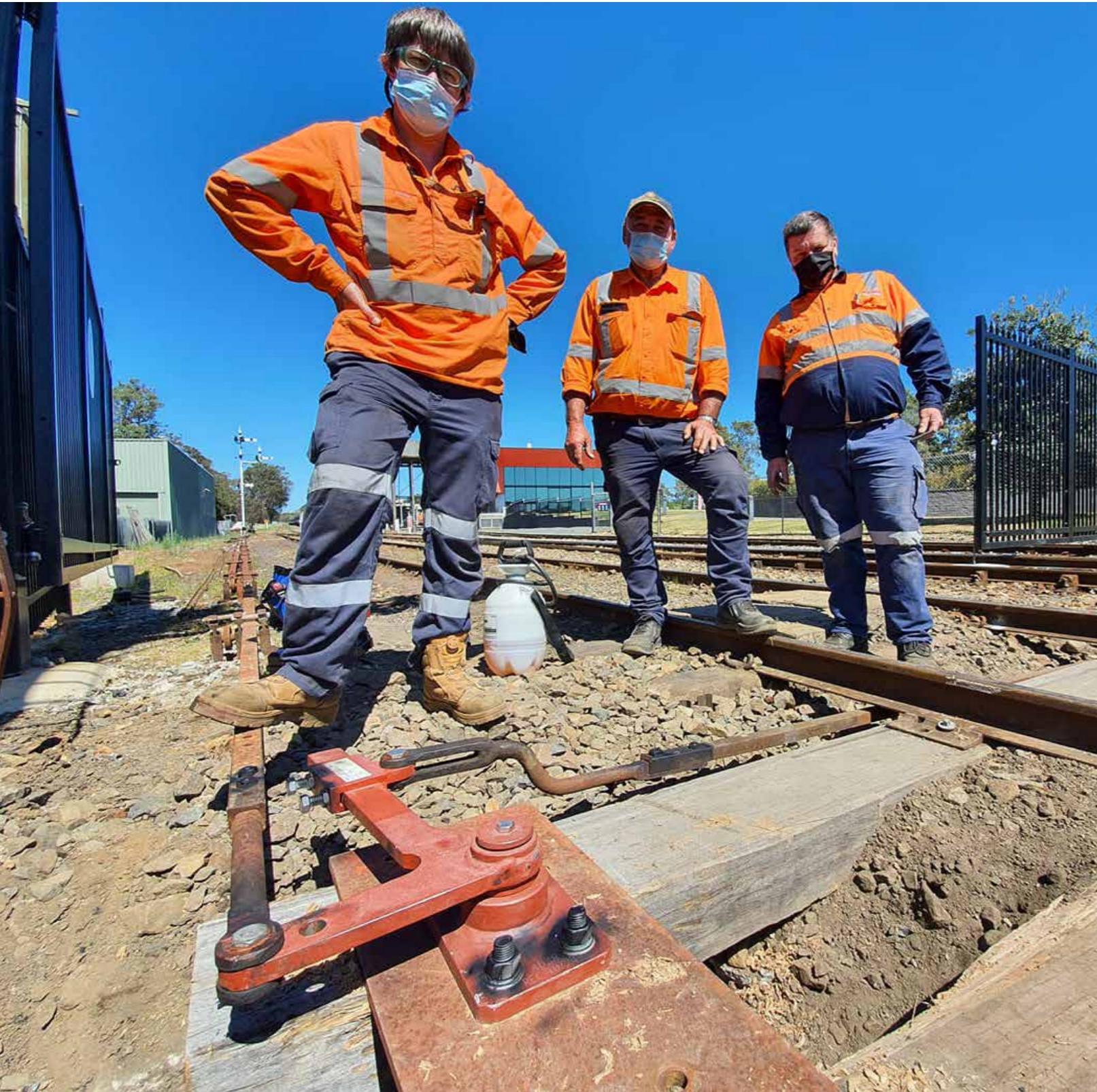
THNSW's Ben Armstrong, Les Kelleher and Peter Lawrence undertake essential work to points on the Loop Line. ▲
